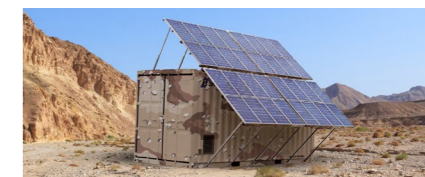
Solar Energy Off-Grid Solution (Shams Station)
